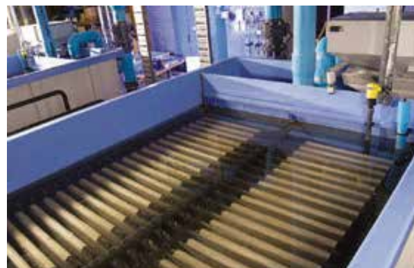
Vacuum DE filters (source: Ian Coombes Ltd)
