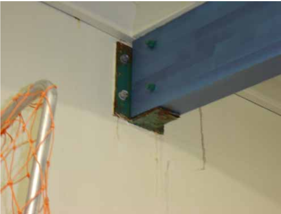
Corroded steel supports.
