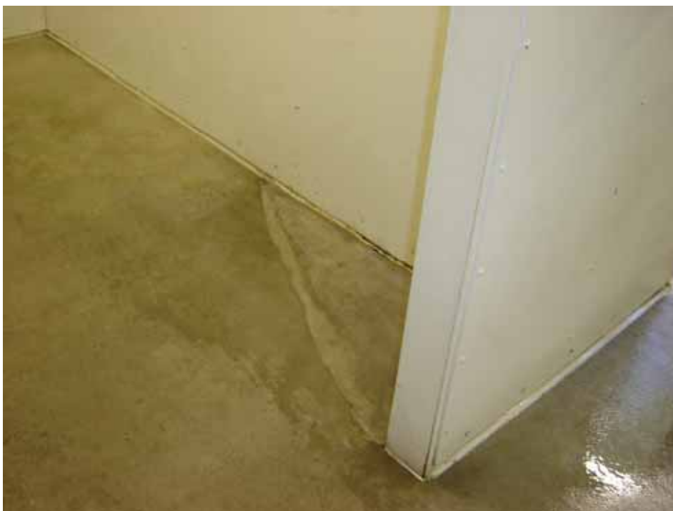
A patch up job on a changing room floor with inadequate slope
