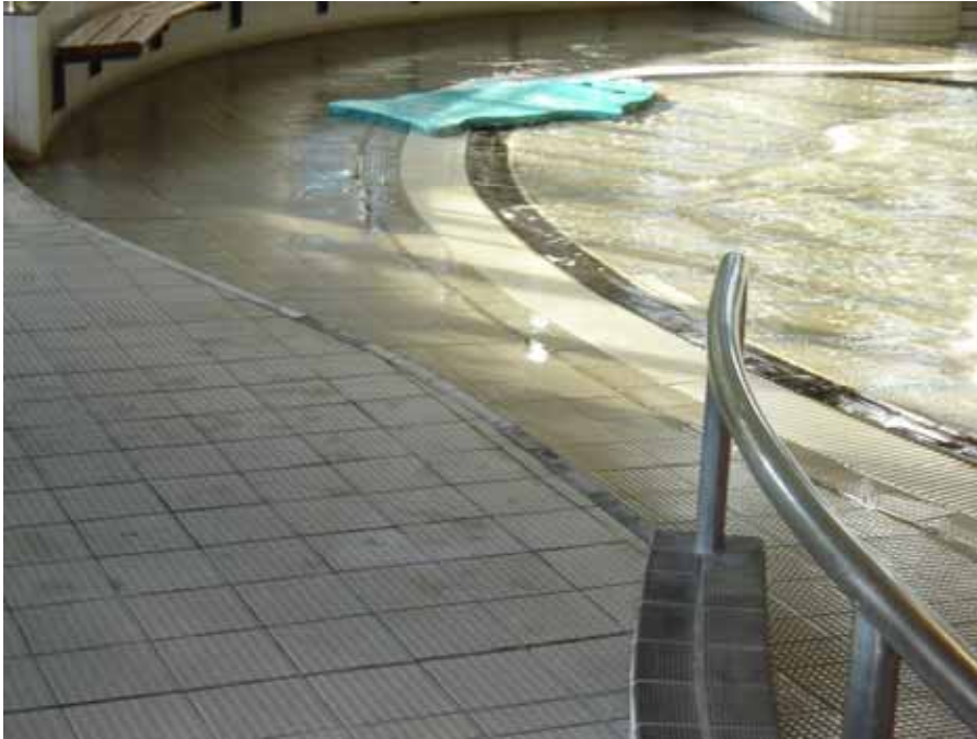
Poolside wash-down water flowing into pool over flow channels
