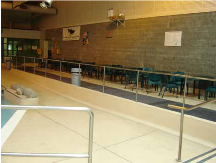
Restricted walkway between hand rail & wall.
