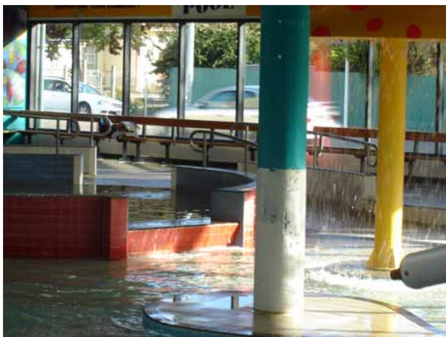
Two examples of high temperature water flowing from the Toddlers' or spa pool to the leisure pool.
