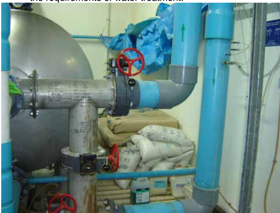
An example of poor provision for chemical storage.
