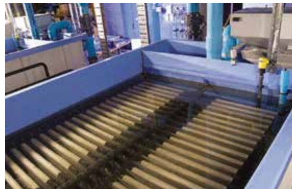
Vacuum DE filters (source: Ian Coombes Ltd)
