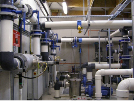
Figure 1: Example of a pool facility plant room
