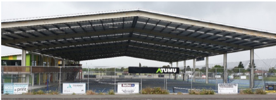
Masterton Netball Centre has a constructed cover with 5.5 metre sides and 7 metre peak. The centre report issues with the rain coming in the sides.
